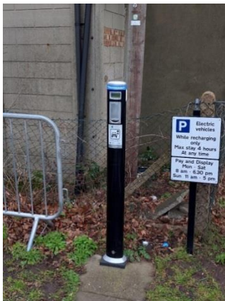
LBRuT 3kw charging point
