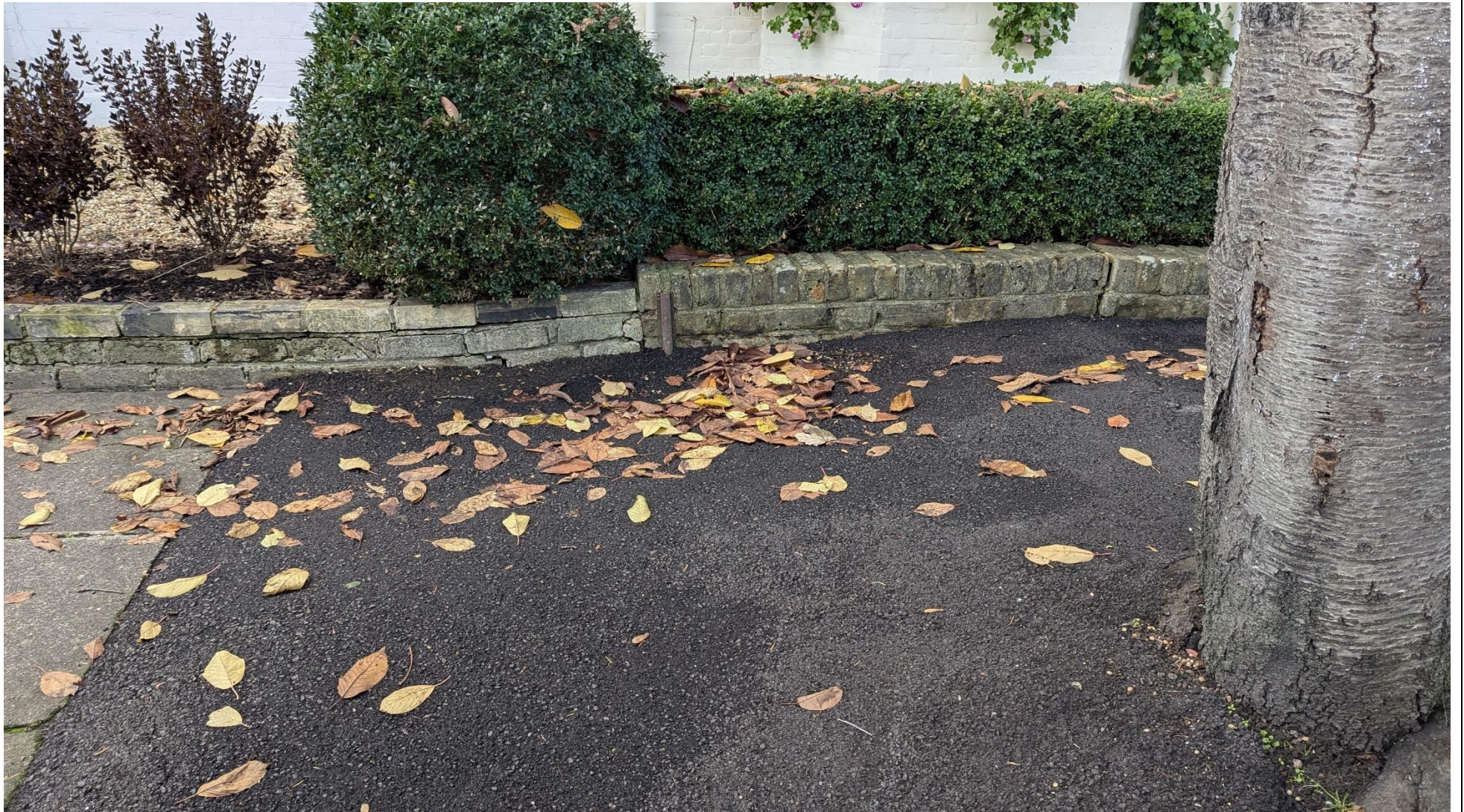
Image 3: Surface tree roots, wall & footway damage
