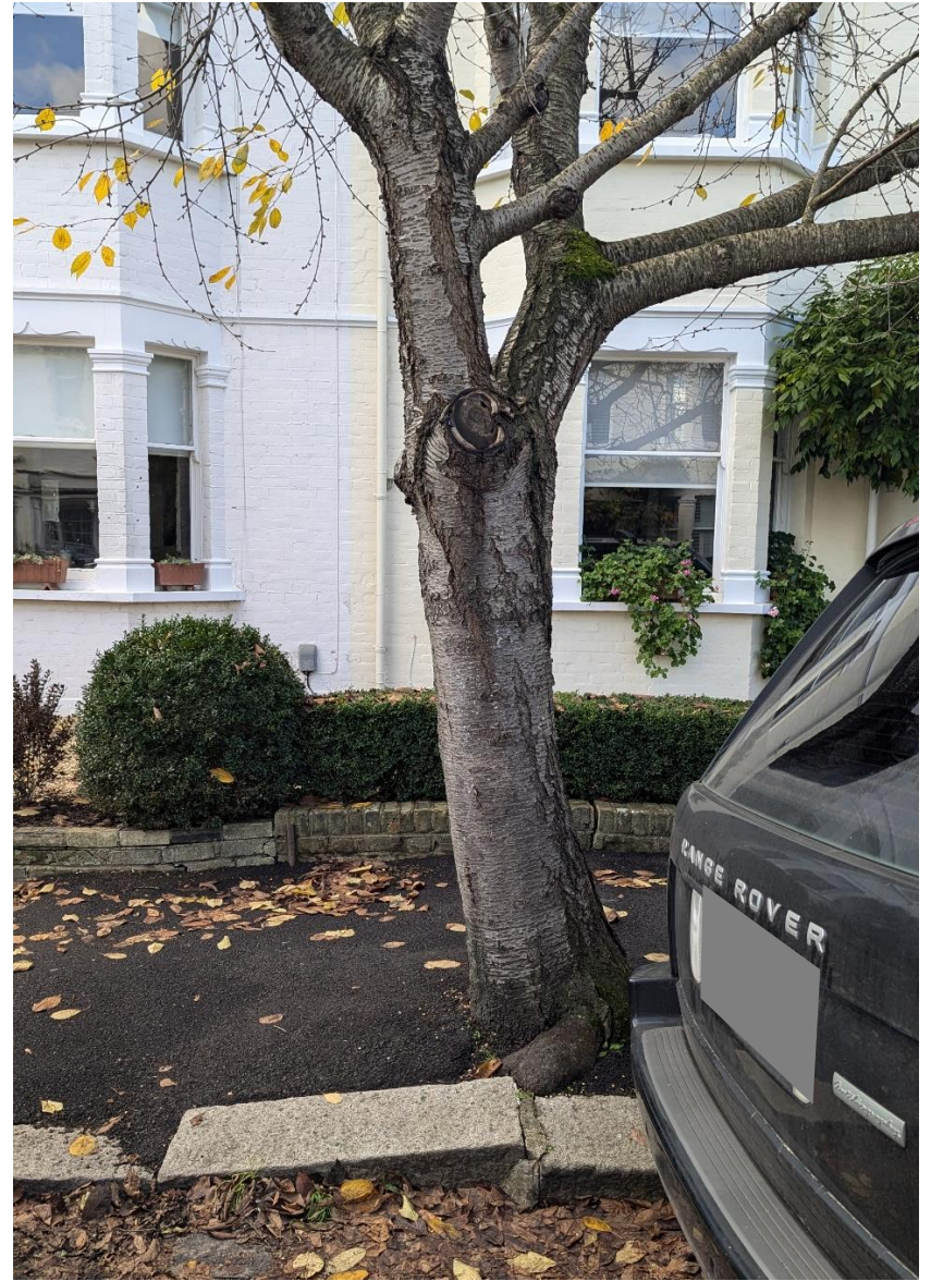
Image 2: Surface tree roots, wall, footway & kerb damage
