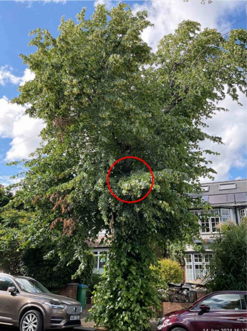
Image shows tree in street scene with location of failed union circled.
