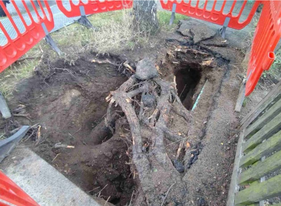
Image shows root damage caused by excavation for maintenance to underground services
