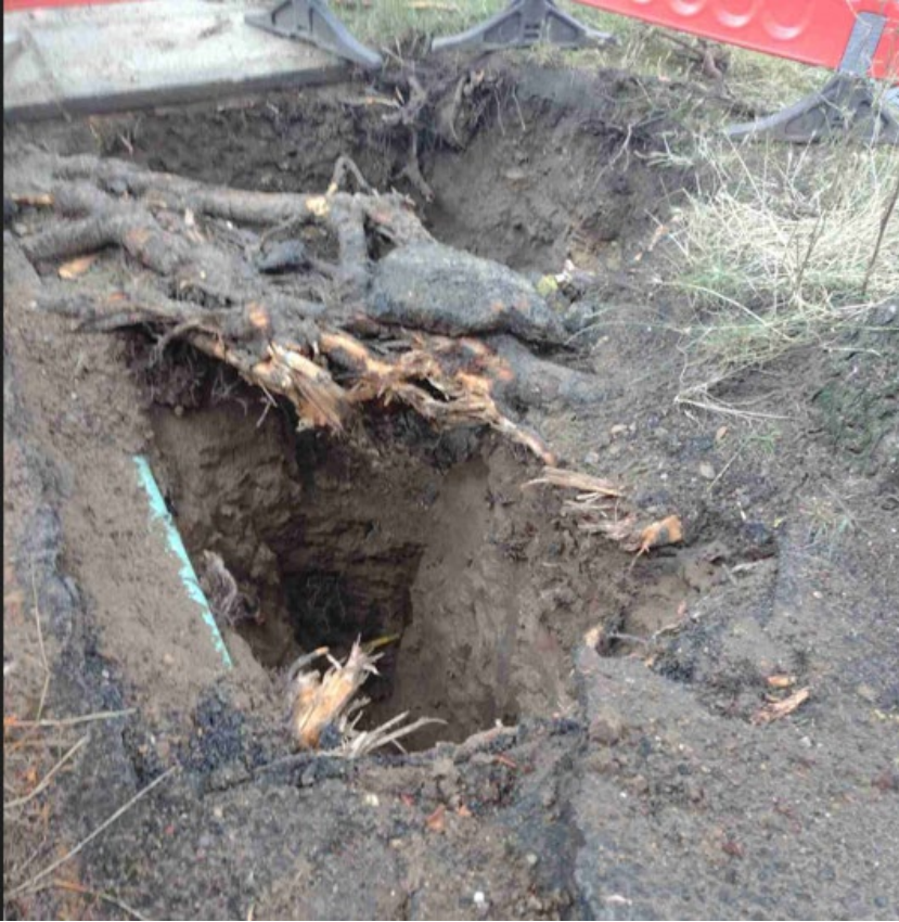
Image shows root damage caused by excavation for maintenance to underground services.
