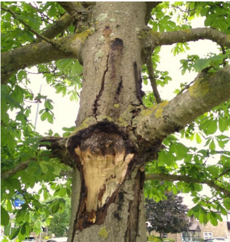
Image shows wound from recent branch failure and bleeding bark canker on upper stem.
