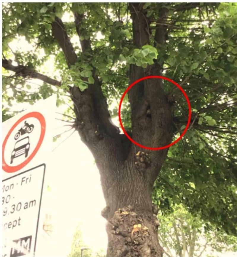
Image shows opening to cavity on stem at crown break circled in red.
