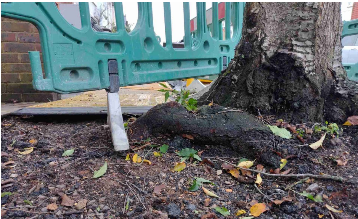
Image shows exposed damage roots at base of trunk obstructing pavement access.
