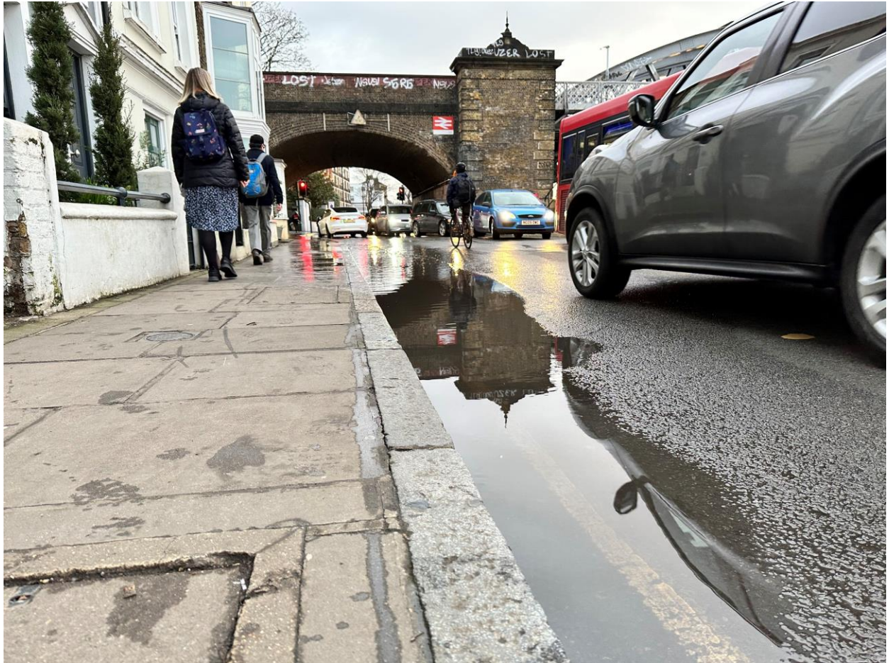
Figure 2-2 Surface water flooding on a road in Richmond (Image source – Richmond LLFA)
