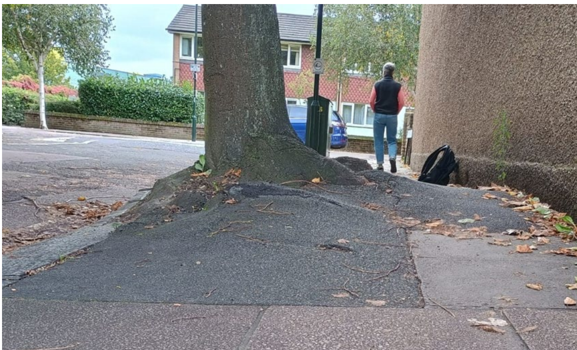
Image shows raised roots causing pavement disruption.
