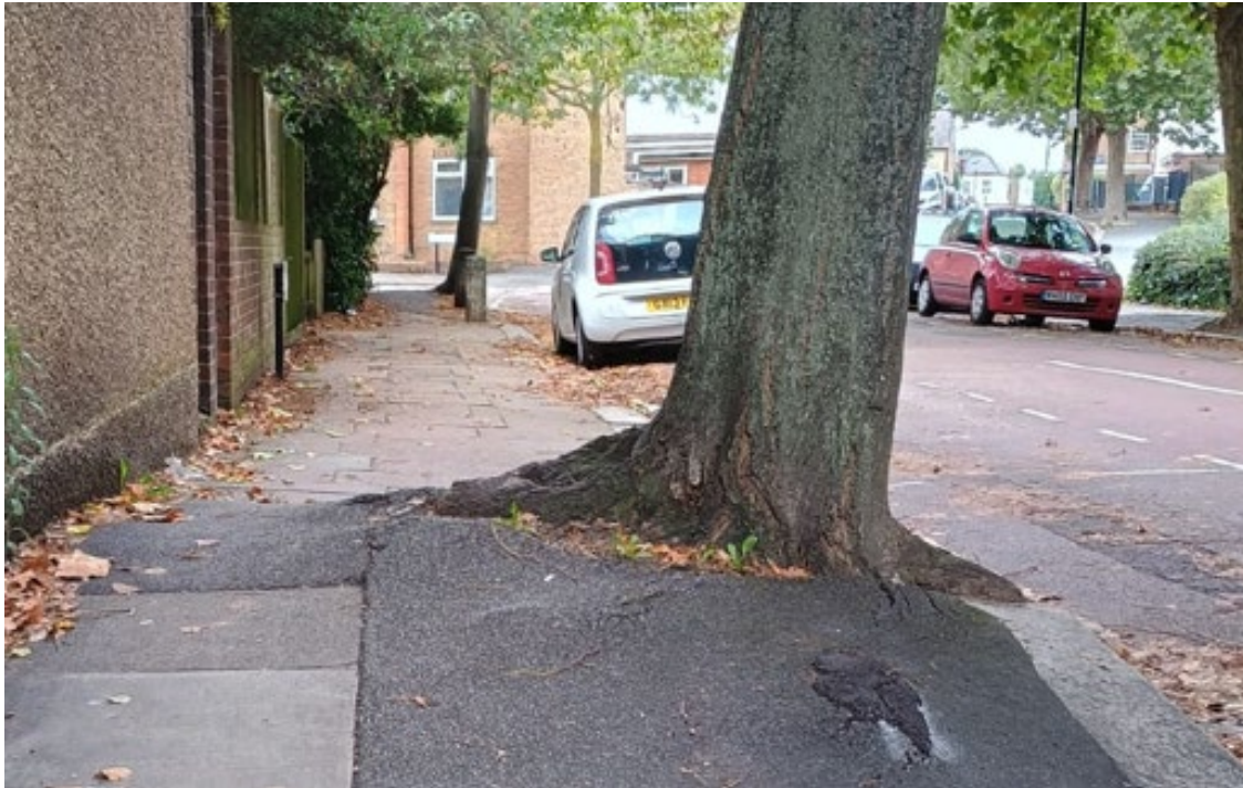
Image shows raised roots causing pavement disruption.
